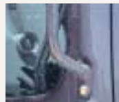
Easily repaired bolted handrails
