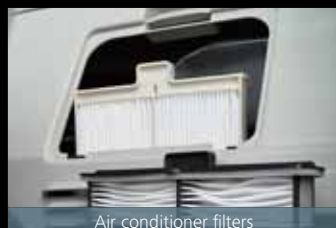
Air conditioner filters
