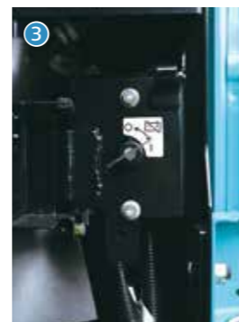
3 Battery shut-off switch
